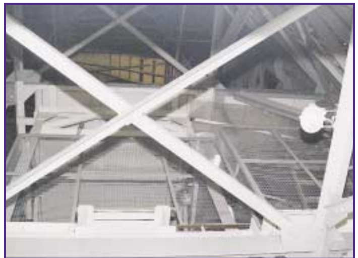
Suspended machine room
