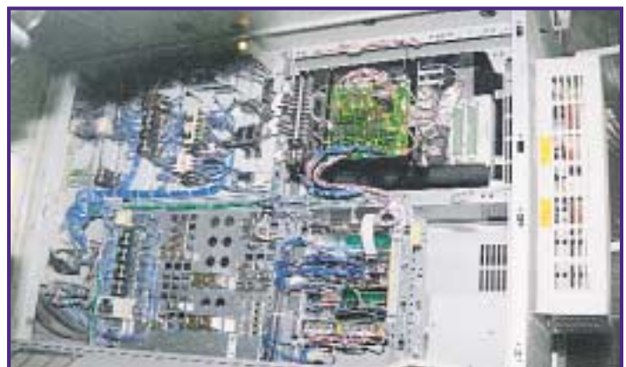
Fujitec up/down selective controller
