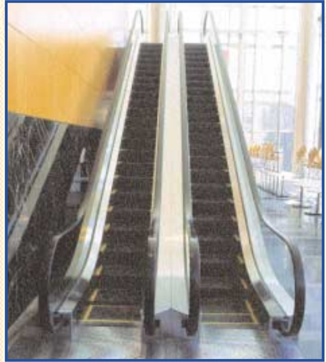
Front view of escalators
