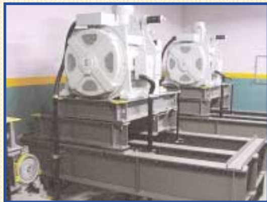
AC gearless machine (high area)
