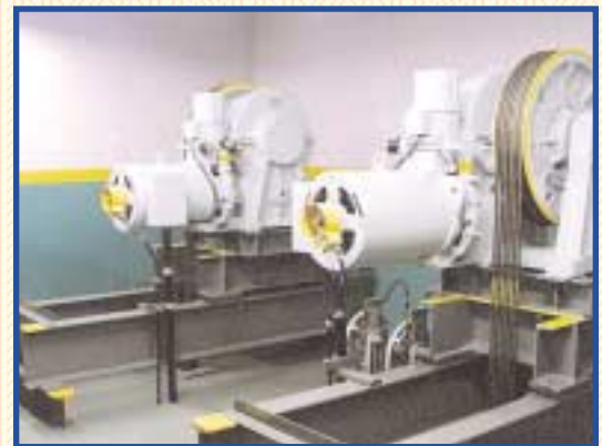
Exceldyne geared machines (low area)
